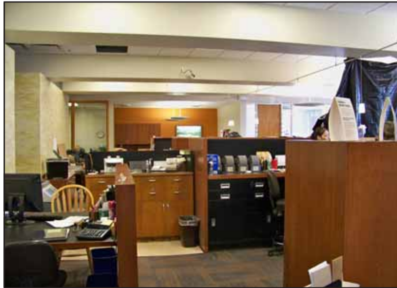
Although entry is still limited to the South door, one can see how the completed lobby will look at the Columbus Junction State Bank. Most of the temporary wall has now been removed, and the new teller counter and lighting fixtures are now very much evident.
