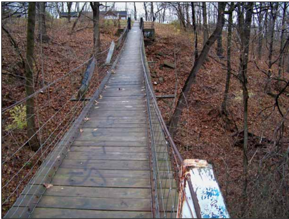
Damaged handrails at the Swinging Bridge
