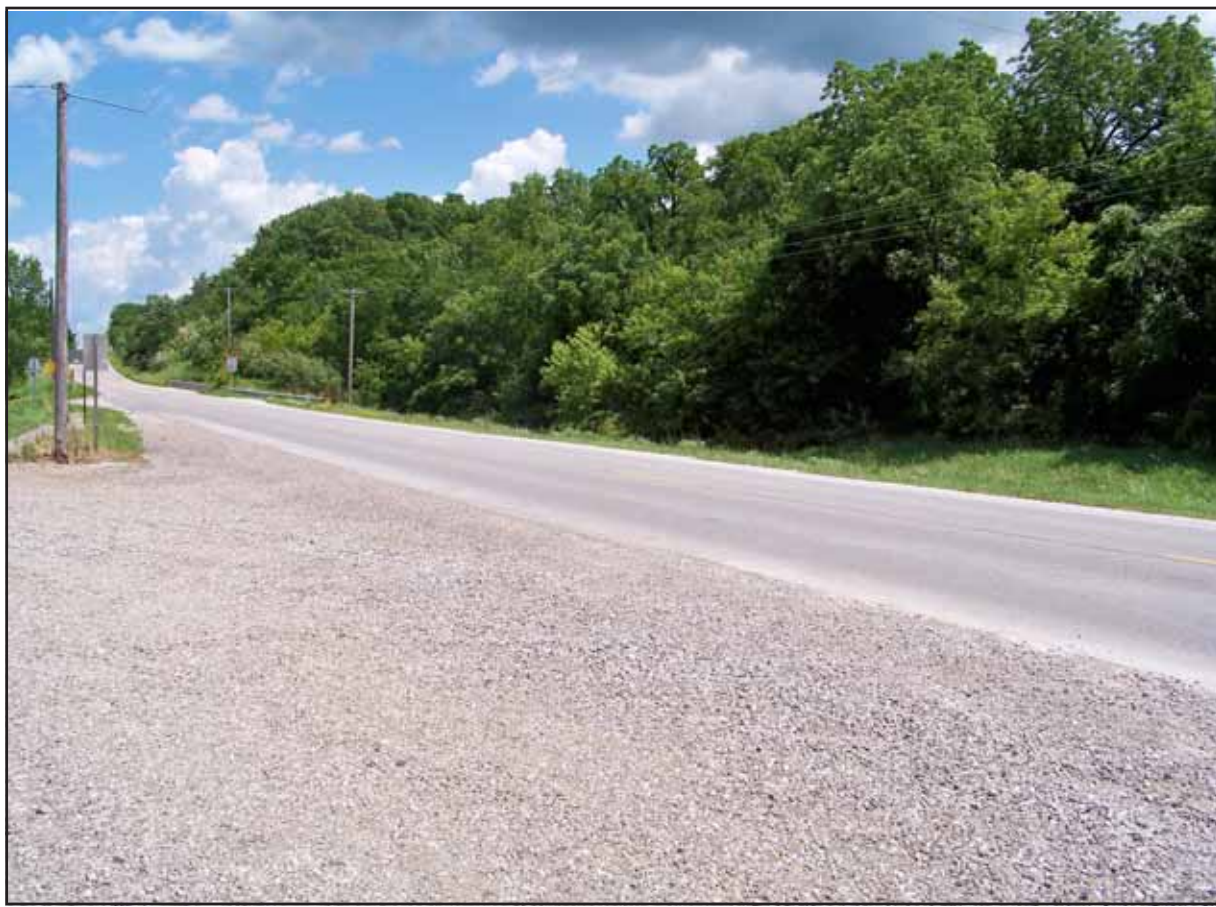
Area on Highway 92 where water overtook two autos during heavy rain.
